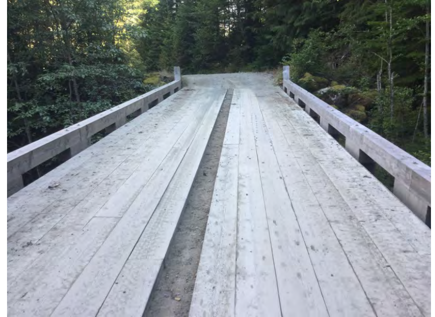
Deck Note Track Marks
