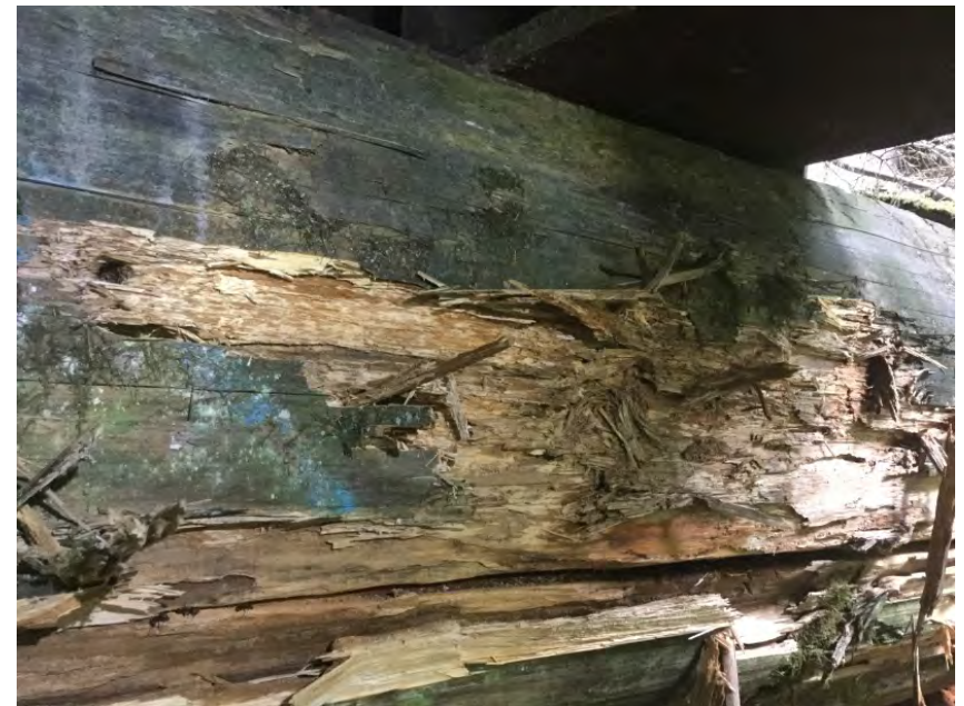
R/B U/S Corner Split in Top Crib Log with Signs of Bug Infestation
