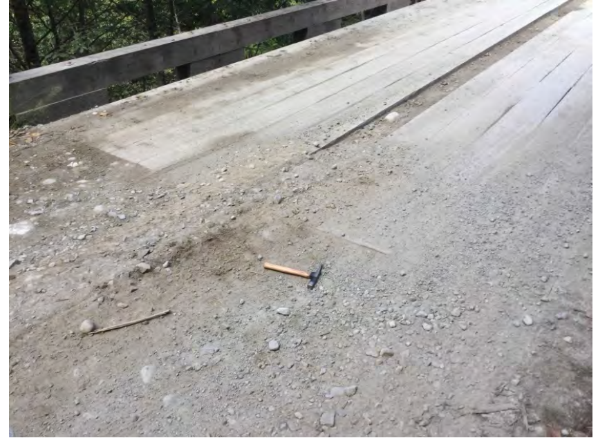
Left Approach Pothole Forming
