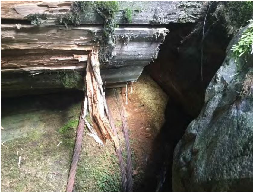
R/B U/S Corner Signs of Bug Infestation in Top Crib Log
